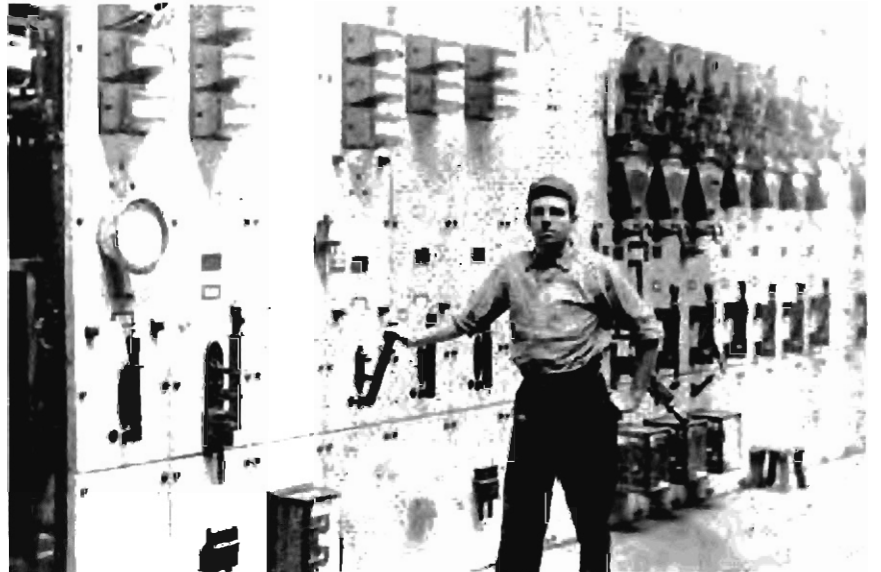
Substation operator William G. Horsch, now of Woodbury, N. J., at the alternating current panel in the Salem rotary station.
